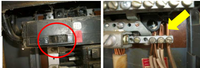
The breaker switch is
